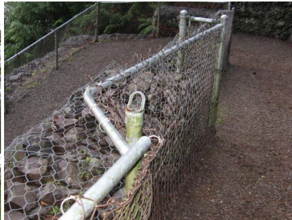
Storm-damaged fence @ Lewis St Park
